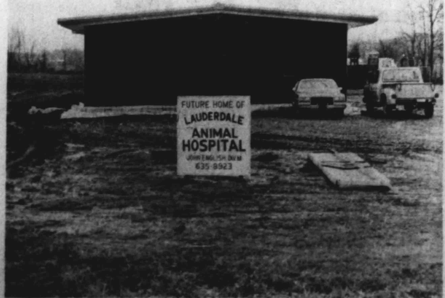
NEW ANIMAL HOSPITAL under construction on Highway 51 By-pass by John English, DVM.
